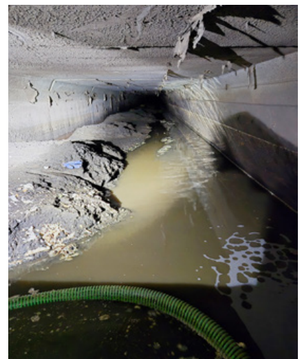
Sediment in culvert beyond the dam
